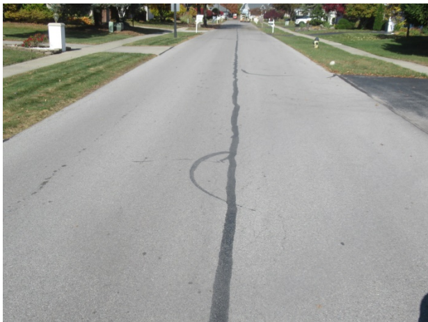
Typical condition of the pavement with crack repairs at the centerline at "Phase III"
