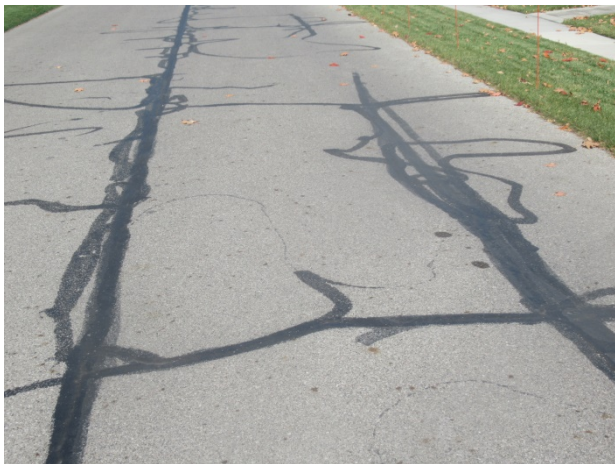
Crack repairs and minor settlement
