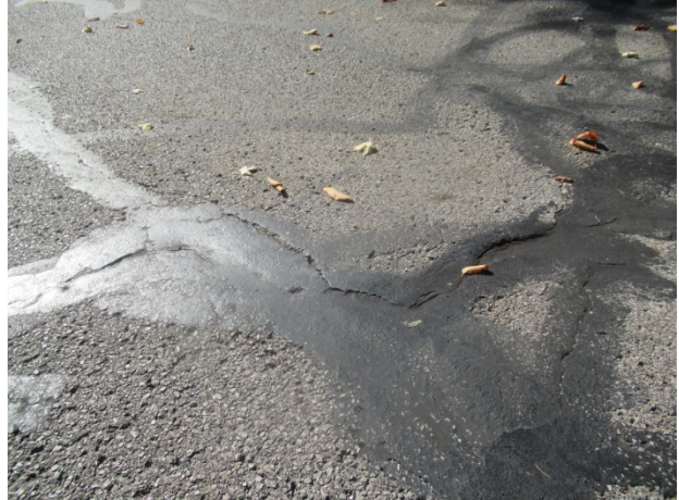
Pavement cracks and settlement at location of previous repair
