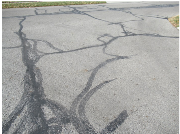
Repairs throughout intersection of East Shoreline Drive and North Moon Lake Drive
