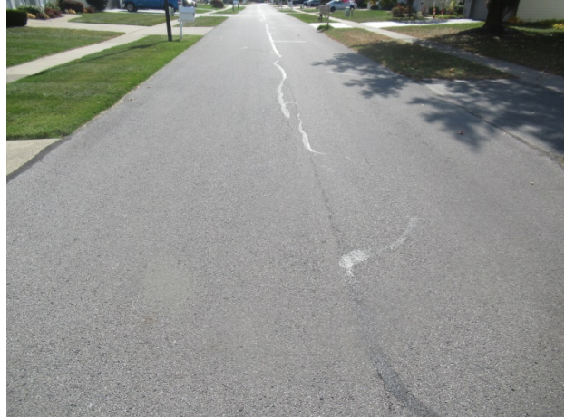
Streets in good condition with minimal cracks and repairs throughout "Phase III"
