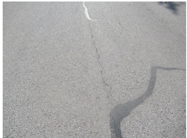
Isolated unrepaired cracks at centerline, Cove Harbour Drive
