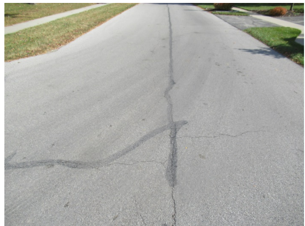
Isolated unrepaired transverse and longitudinal cracks
