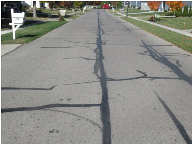
Crowned street pavement with previous crack repairs at East Shoreline Drive
