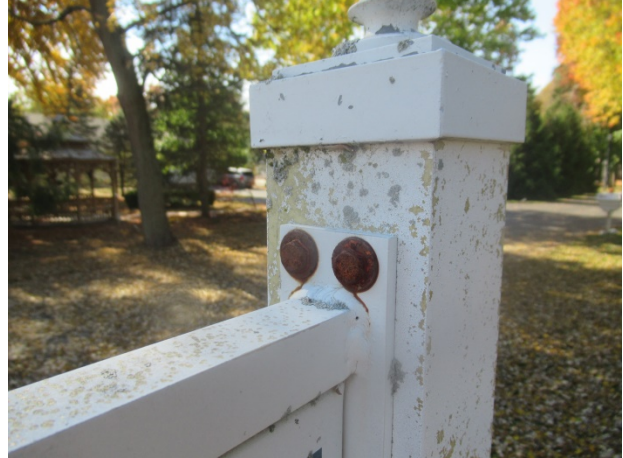
Rust at fasteners and finish deterioration
