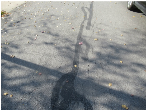
Isolated instance of high frequency of longitudinal cracks, Hidden Forest Drive
