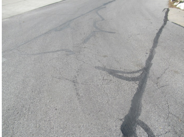
Isolated instance of widespread deterioration at intersection of North Shoreline Drive and Cove Harbour Drive
