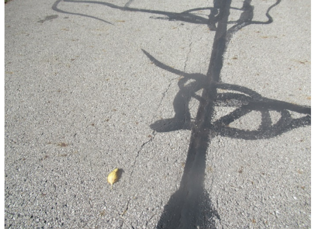
Unrepaired cracks adjacent to repaired cracks at North Moon Lake Drive
