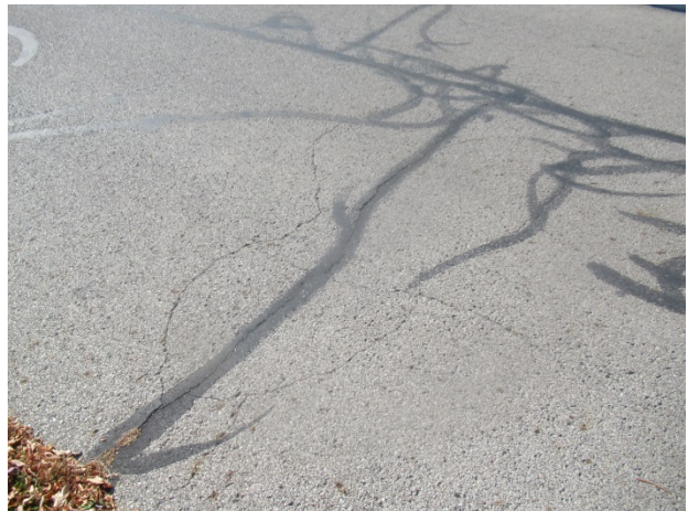
Isolated instance of unrepaired cracks at East Shoreline Drive
