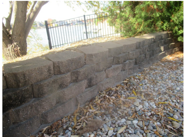
Retaining wall deflection
