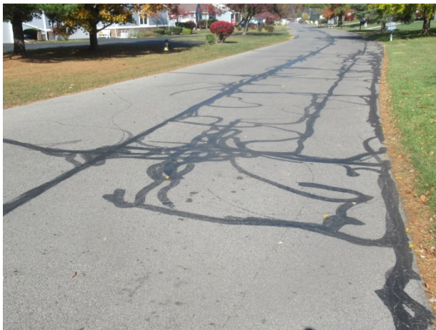
Repaired cracks throughout the shared pavement at East Shoreline Drive
