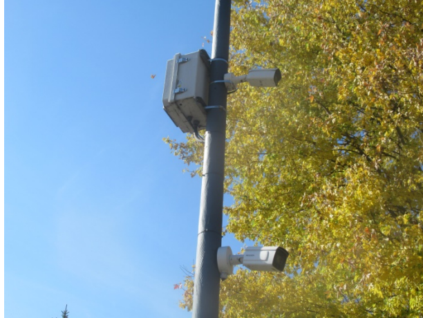
Security cameras mounted to the light poles
